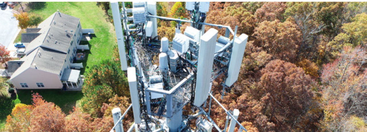
HARMONY TELECOMMUNICATIONS TOWER Ohio, USA Partner: Ardian
